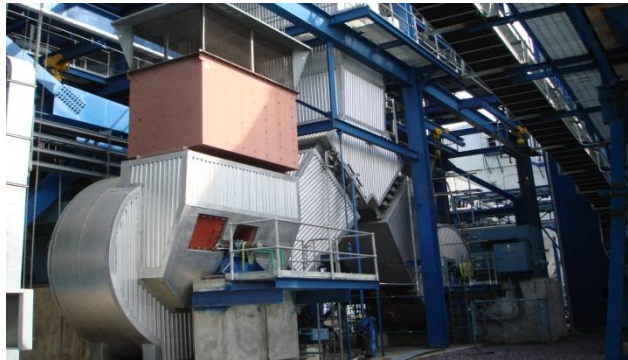
Gambar.2.8 Primary Air Fan
